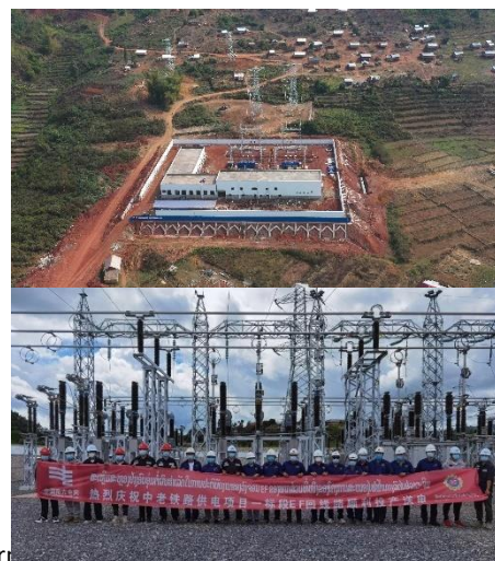
Power Supply Project for Laos-China Railway, transmission BOT project, Laos. 20 cct 115kV T/Ls, construction complete March 2021.
